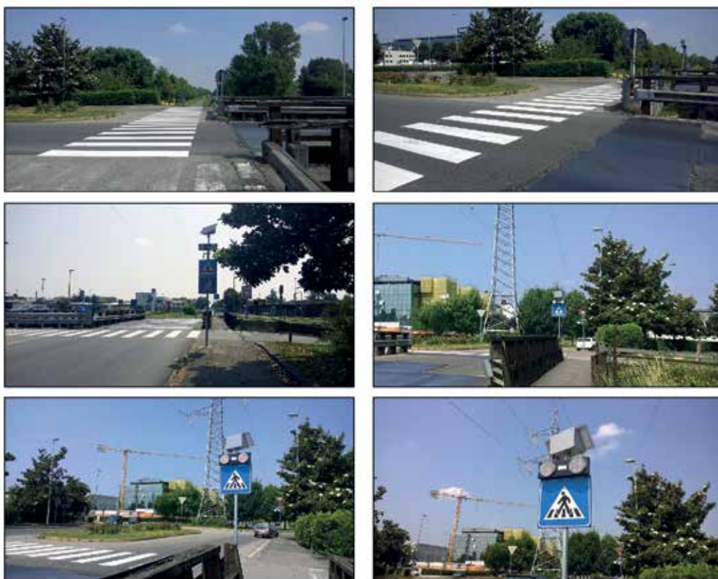
picture 15 Photos of the completed interventions for improving cycling safety conditions in the project junction. From top to bottom: - the zebra crossing reconnecting Naviglio Pavese bike path; - the vertical road signs highlighting the presence of the cycling crossing; - the flashing lights making the crossing more visible to car drivers.
